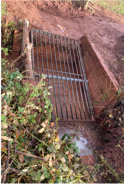
Cleared out debris screen
