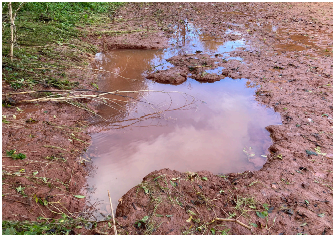
Hole created by culvert B outflow
